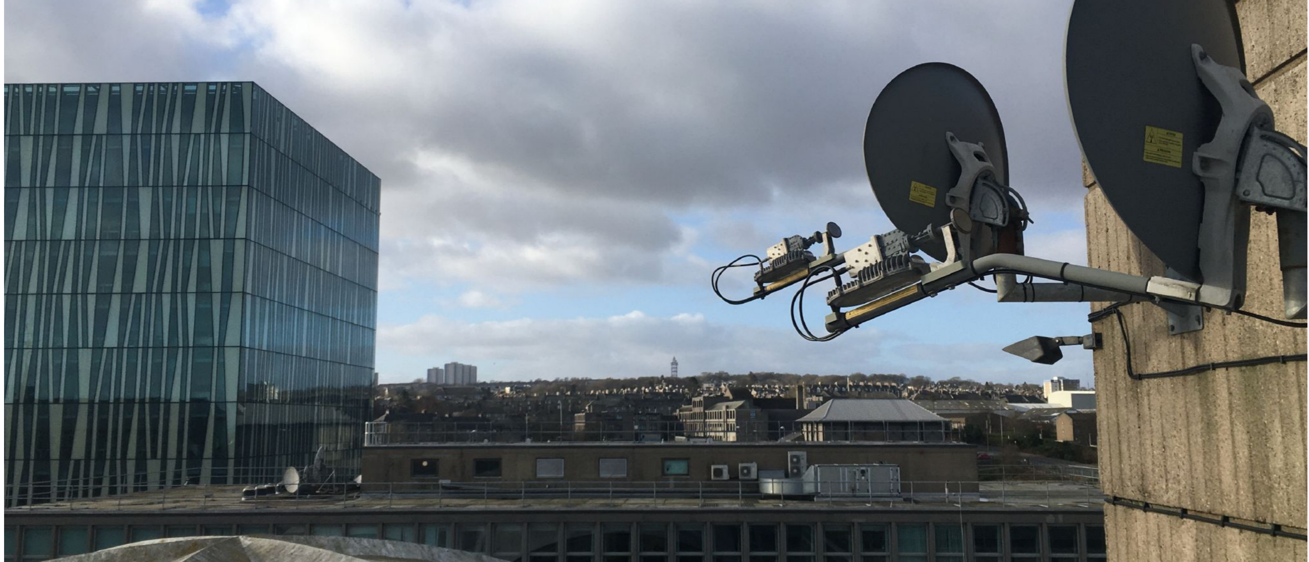
Our KA Band satellite dishes that connect to the HYLAS 1 satellite looking over the noted Sir Duncan Rice library building at the University of Aberdeen.
