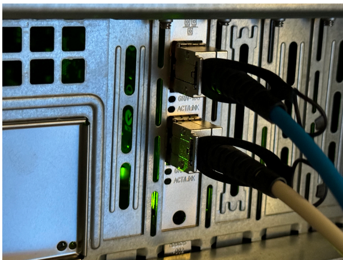
Intel X710-DA2 SFP+ Ports with DAC Cables Attached
